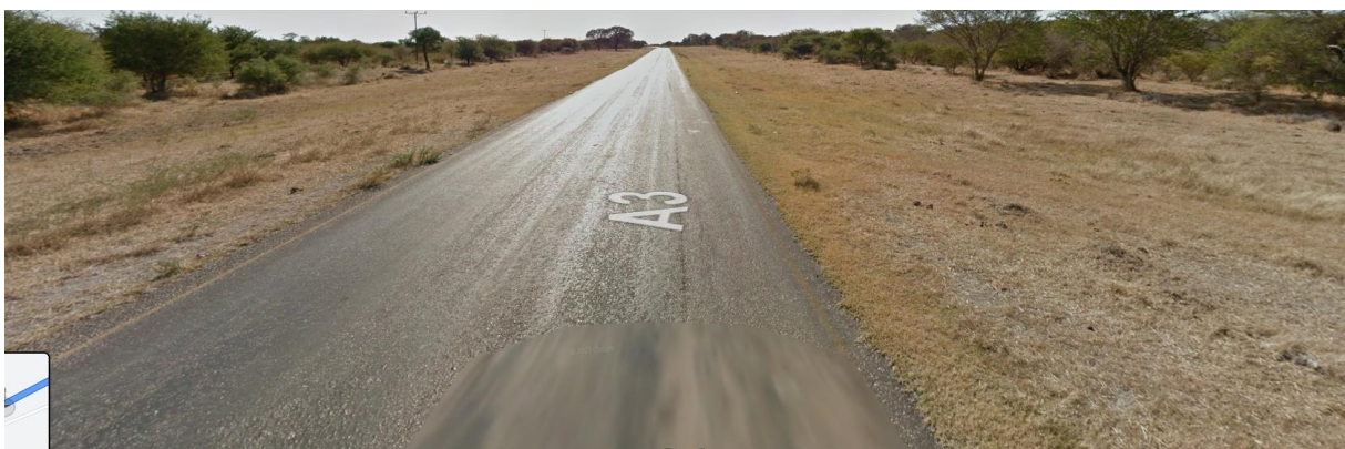
Figure 15: Road condition from Toteng to Maun 96
