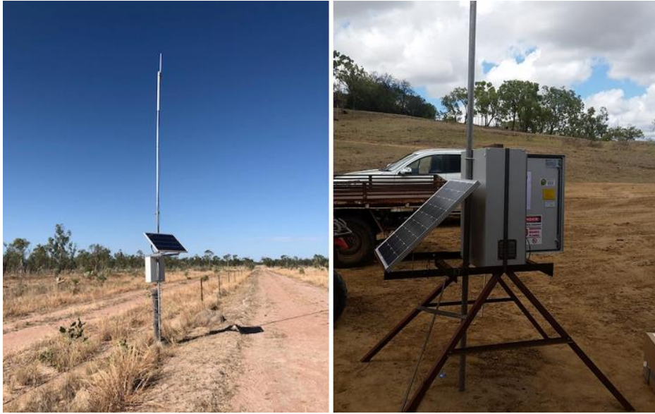
Figure 17: LoRa off-grid antennas 102
