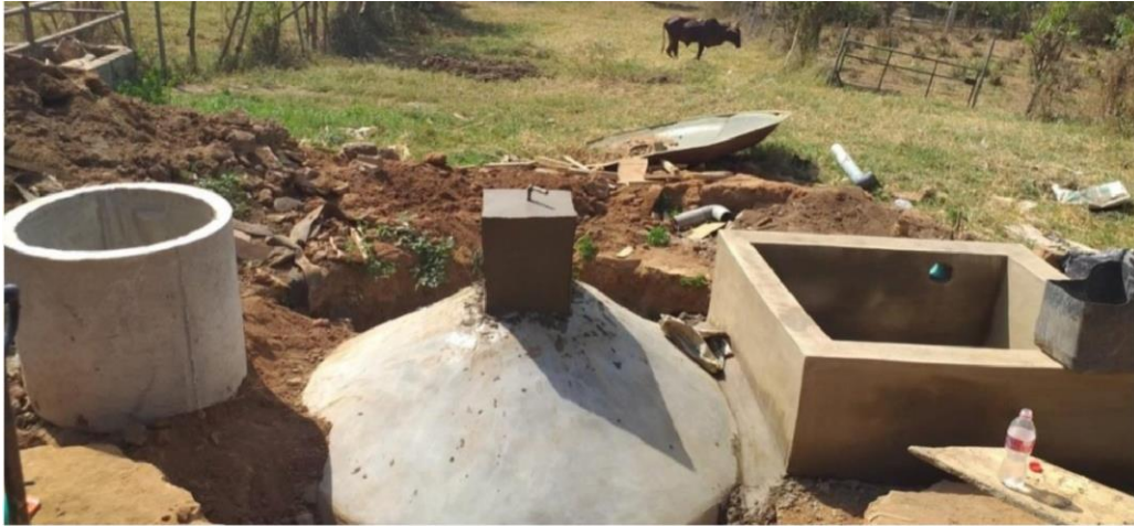
Figure 9: Completed digester, pilot project in Ibadan, Nigeria 61
